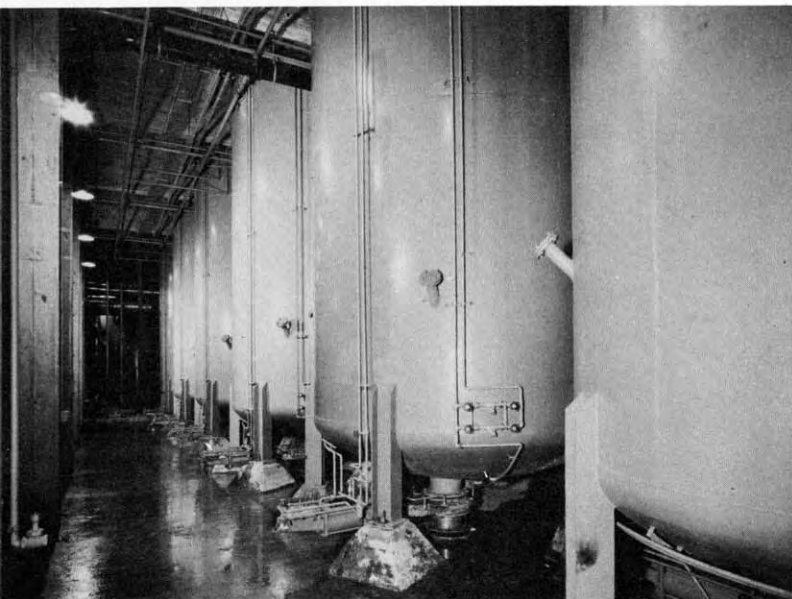
Battery of six tile-lined bleach cells, each with 7½ tons pulp capacity.
