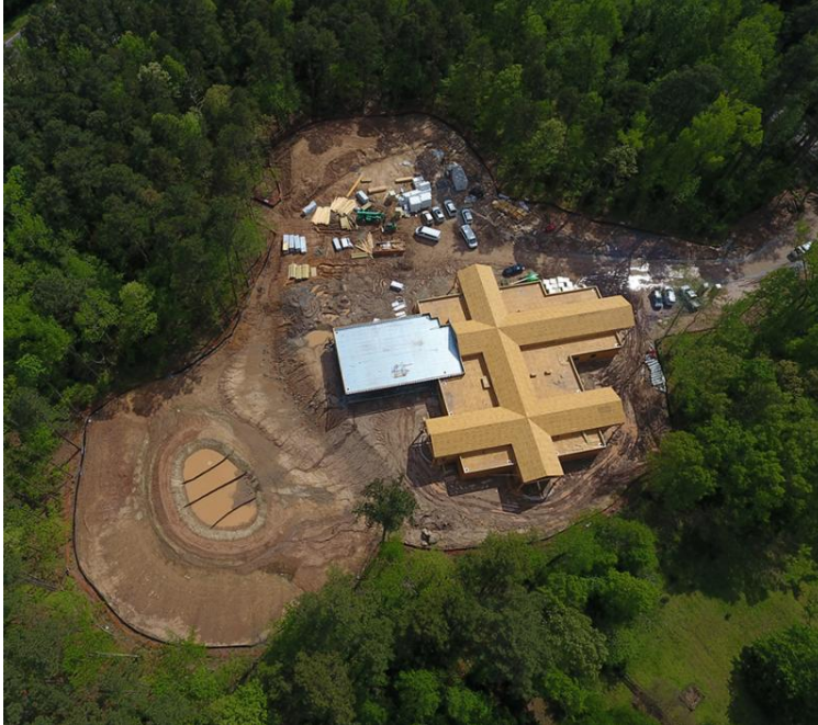
The building as of April 27. The metal section on the left will house the archives.
