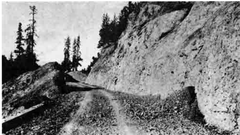
These photos taken by Norcross in July, 1926 show major road construction in a section of the Applegate Road. left: a section looking "approximately" south; below: the same cut looking "approximately" north.
