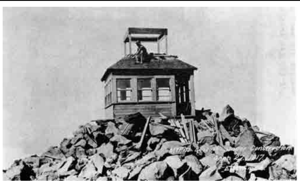
Mt. McLoughlin Lookout house under construction by Lookoutman Jenns, Sept. 27, 1917. Construction was completed in October. - Photo by E. W. Smith
