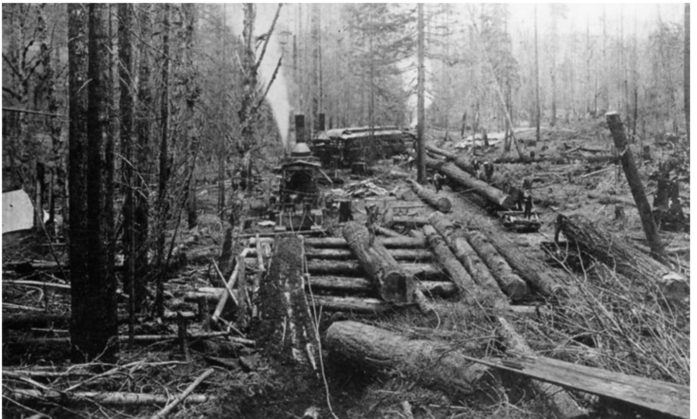
In the Oregon woods, it is often cheaper to put a railroad on stilts (piles and trestles) than to excavate a roadbed for its track. Notice in the picture the giant size of some logs in the center. The machines in the picture are pile drivers and donkeys.
